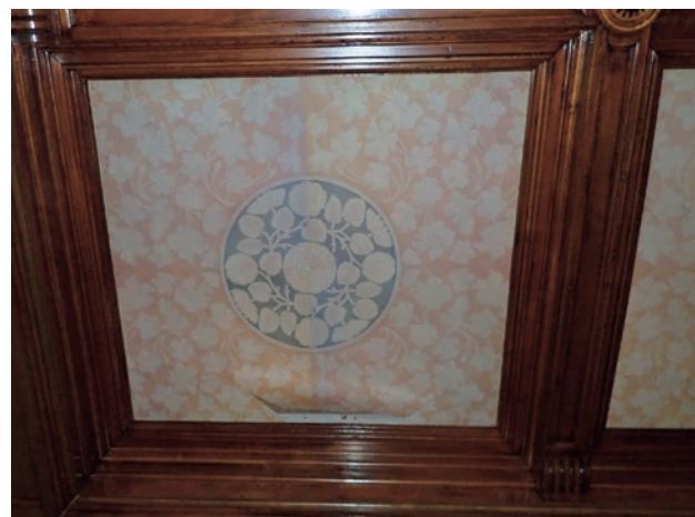
photo Deteriorated ceiling paper in the sales room
