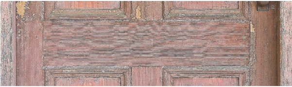
photo 8 Main building front door (before repair)
