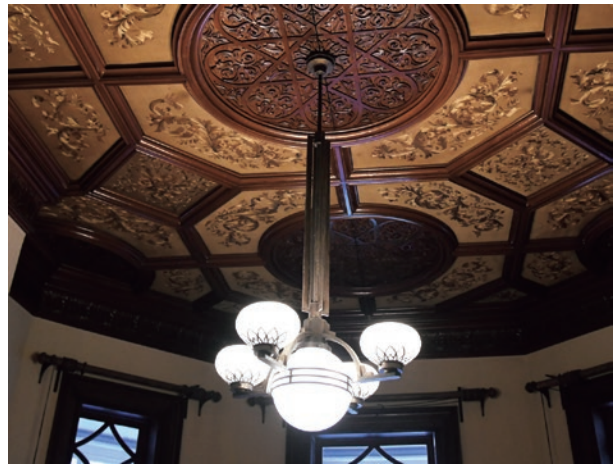
photo Original pendant light in the lady's guest room on the 1st floor
