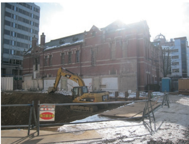
photo 6 North outer wall before conservation (photographed in 2012)
