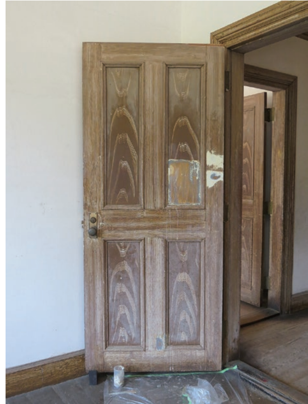
photo 3 Main building No. 4 room door peeling investigation status
