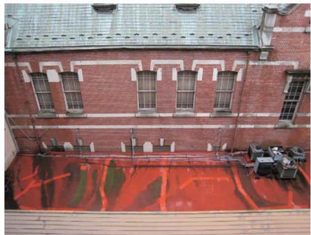
photo 5 North outer wall before conservation (photographed in 2008)
