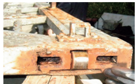
photo app.2-3 Corrosion of rail support
