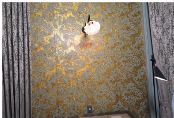
photo Restored wallpaper of the small guest room (southeast room) on the 2nd floor
