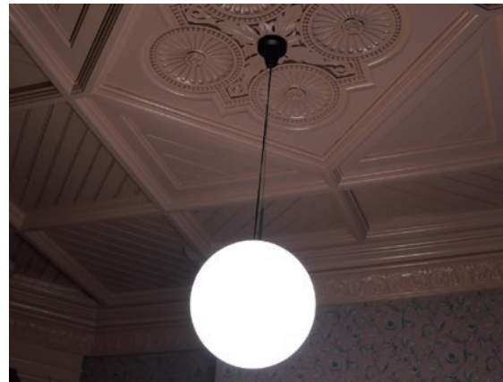
photo Commercial pendant light in the arge guest room on the 2nd floor
