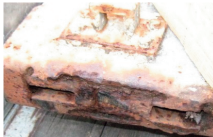
photo app.2-2 Corrosion of rail
