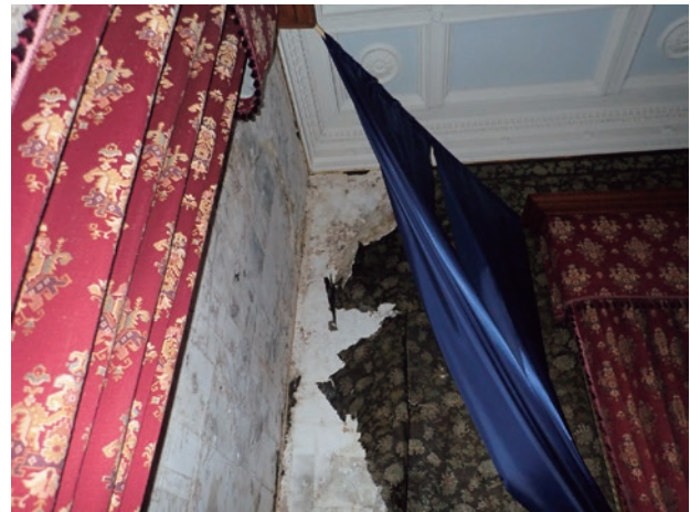
photo Wallpaper that is currently peeling off
