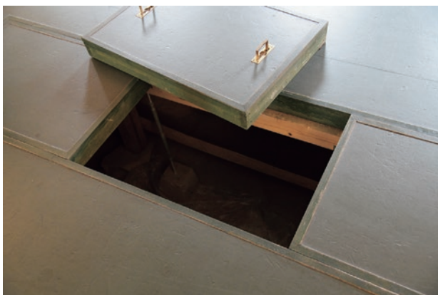
photo Underfloor space, Air-conditioning facilities and others are concentrated here
