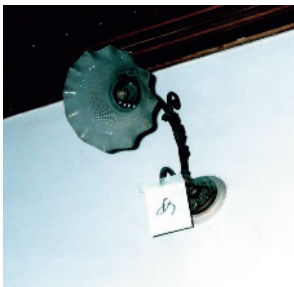
photo app.2-33 West stairs: damaged lamp
