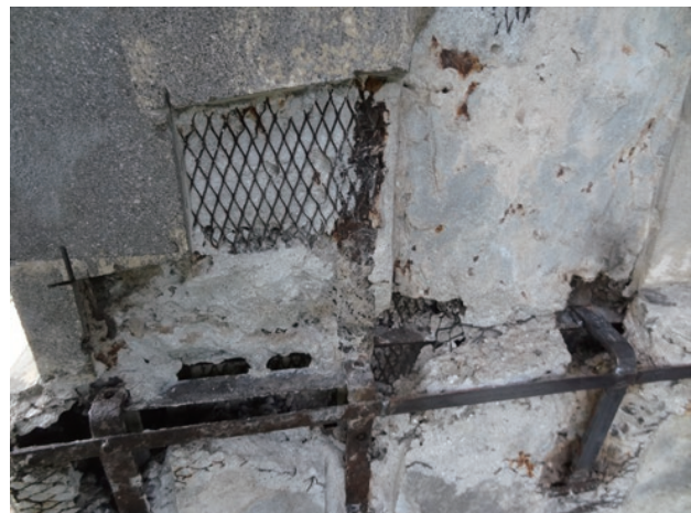
photo 3 The original diamond-shaped metal lath and steel frame members, after removal of damaged mortar finish
