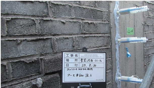
photo 5-6: Injecting cement slurry under low pressure (External wall) (photo provided by : Shimizu Corporation Hiroshima Branch)
