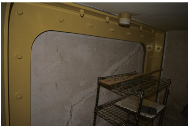
photo 16 Reinforcement with gate-shaped steel framework (in an area not open to the public)
