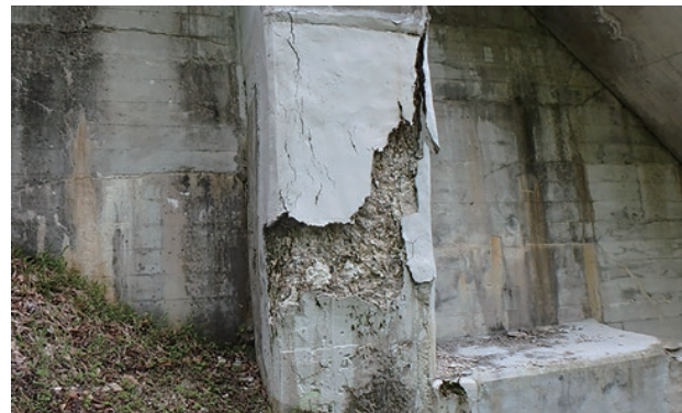
photo 3-3: A buttress deteriorated due to freeze-thaw cycles (the surface coating provided in the past repair project peeled off) (photo provided by : Tokyo Electric Power Company Holdings, Incorporated)
