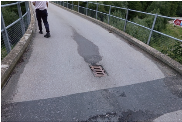
photo 3 Water drainage system on the bridge surface (a catch-basin was provided at the center of the road at each end of the bridge) and newly installed steel railings
