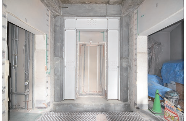
photo 5-16: Sub-entrance reinforced with steel frames (photo provided by : The Japanese Association for Conservation of Architectural Monuments)
