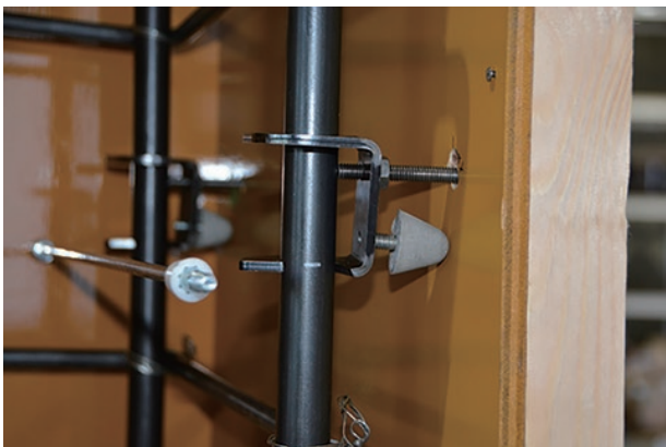
photo 2-5: Separator-pulling devices with spacers installed on a test specimen (photo provided by : The Japanese Association for Conservation of Architectural Monuments)
