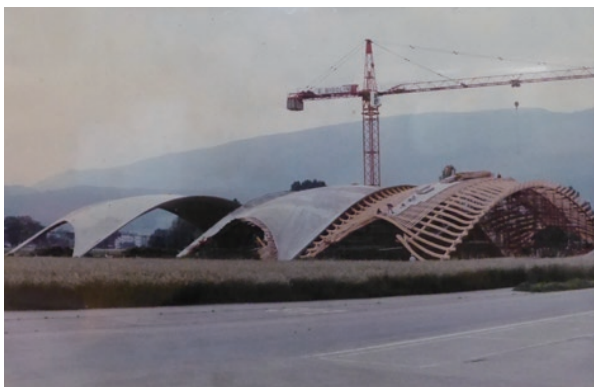
photo 54 Concrete shell under construction (cited from a photograph of a signboard installed on site)
