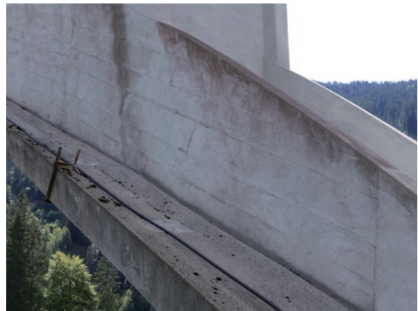
photo 38 Discoloration of the north-side arch ring's concrete
