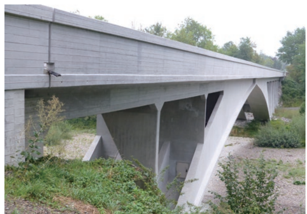
photo 23 Drainpipe protruding from wall balustrade
