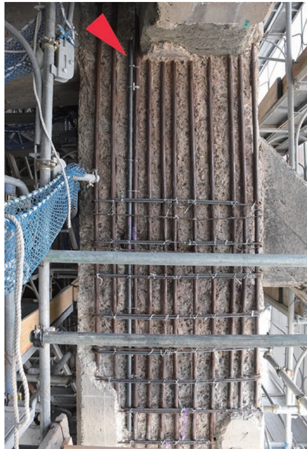
photo 2-7: Addition of a splint (indicated by a red arrow) alongside the corroded bar (photo provided by : The Japanese Association for Conservation of Architectural Monuments)
