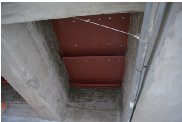
photo 6-8: The space between the steel plates and the existing concrete was filled with grout
