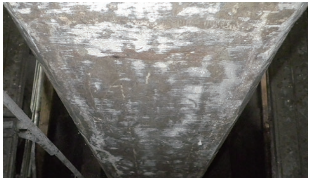
photo 7-5: Appearance after removal of the re-alkalization setup (photo provided by : West Japan Railway Company)
