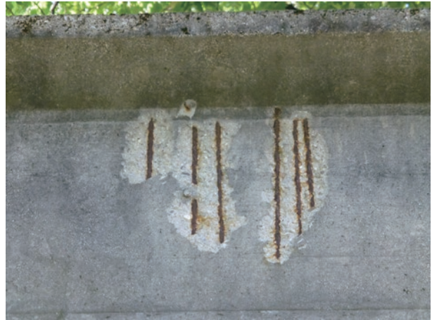
photo 66 Corroded steel bars (1)
