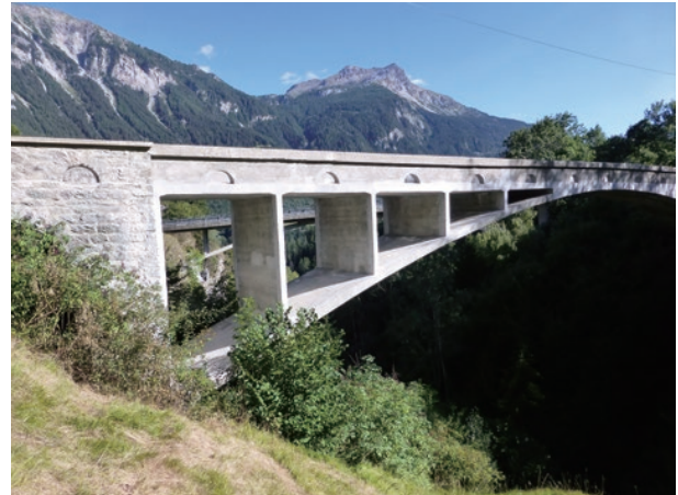
photo 42 Valtschiel Bridge (close view) (cited from a photograph of a signboard installed on site)
