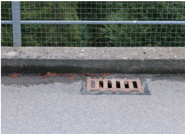
photo 13 Catch-basin of the Schwandbach Bridge (at the edge of the inner curved side near the center of the bridge)
