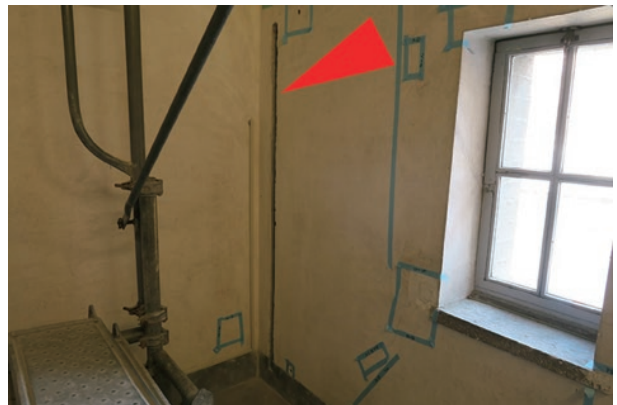
photo 5-17: A seismic isolation slits provided in an anteroom wall (indicated by a red arrow)
