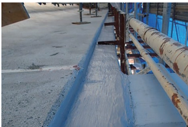
photo 3-5: Protective film applied over the whole concrete surface of the crest (photo provided by : Tokyo Electric Power Company Holdings, Incorporated)
