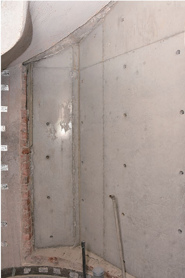
photo 5-14: RC wall of staircase after reinforcement (photo provided by : The Japanese Association for Conservation of Architectural Monuments)
