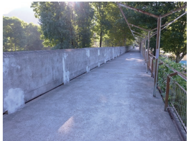
photo 62 Repaired concrete balustrade wall (the color of the concrete repair is conspicuously lighter)
