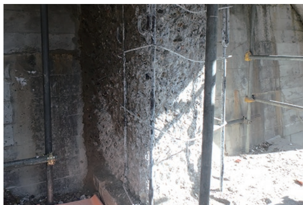
photo 3-8 : Deteriorated concrete chipped off and the exposed concrete surface cleaned (photo provided by : Tokyo Electric Power Company Holdings, Incorporated)
