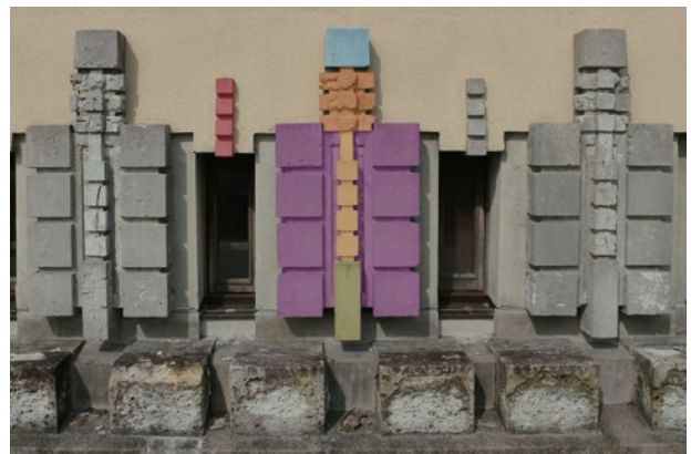
photo 1-4 : All five separate parts of a type B artificial-stone ornament were reassembled (They are color-coded) (photo provided by : Architectural Research Association)
