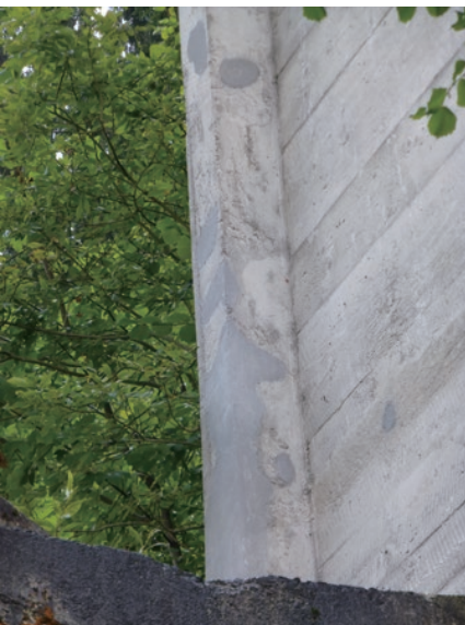
photo 7 Repaired spandrel wall (There is not much difference in color between the concrete used for the repair and the original structure.)
