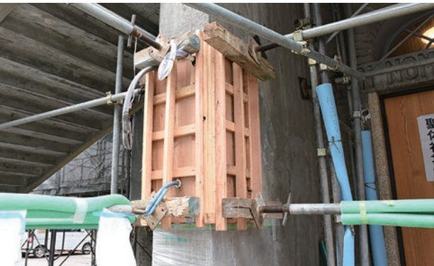
photo 5-12: Refurbishment using the injection method (photo provided by : The Japanese Association for Conservation of Architectural Monuments)
