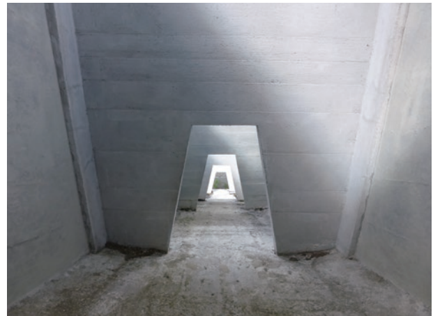
photo 36 Drainage system inside the arch ring
