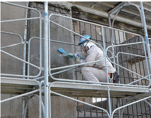
photo 2-2: Cleaning of the concrete surfaces (photo provided by : The Japanese Association for Conservation of Architectural Monuments)
