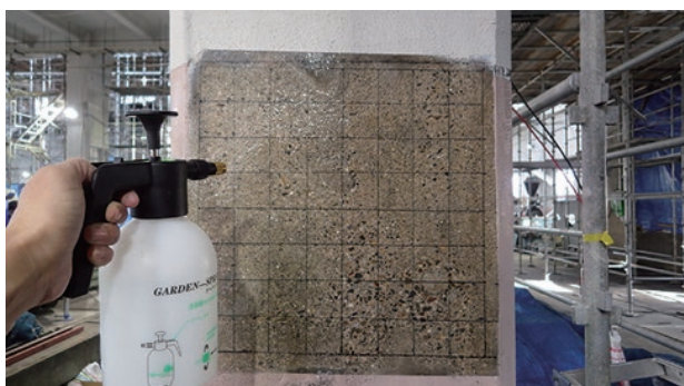
photo 7-7: Water being sprayed before monitoring (photo provided by : West Japan Railway Company)
