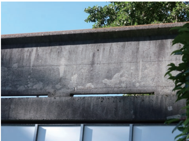
photo 65 The color of the repaired areas is close to the color of the original structure, making them look more natural.)
