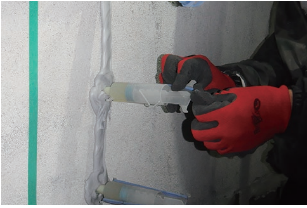
photo 5-3: Injecting epoxy resin under low pressure (Ceiling of the inner sanctum) (photo provided by : Shimizu Corporation Hiroshima Branch)
