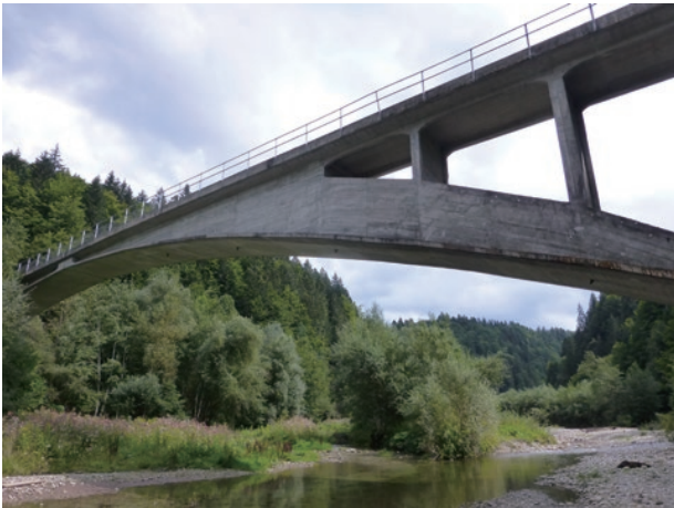
photo 6 The bottom surface of the arch ring was repaired (The traces of annual tree rings left by the timber formwork were reproduced on the surface of the repaired concrete.)
