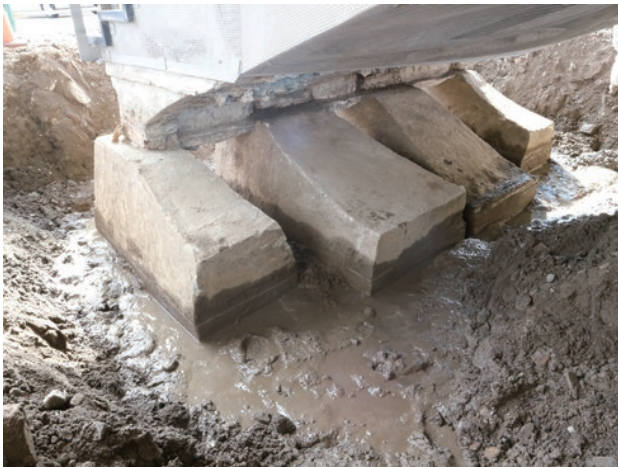
photo 19 Independent foundations underneath the staircase were removed following permission for alteration of the present state.
