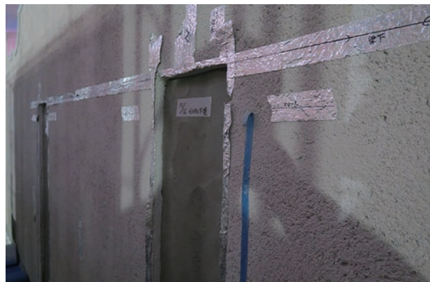
photo 5-18: Seismic isolation slits provided in the main altar (The slits are now being mortared. They will be finally finished so the installation will not be exposed to view.)
