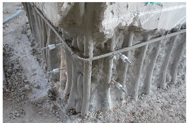
photo 2-4: Mini-cones installed in areas to be repaired (photo provided by : The Japanese Association for Conservation of Architectural Monuments)
