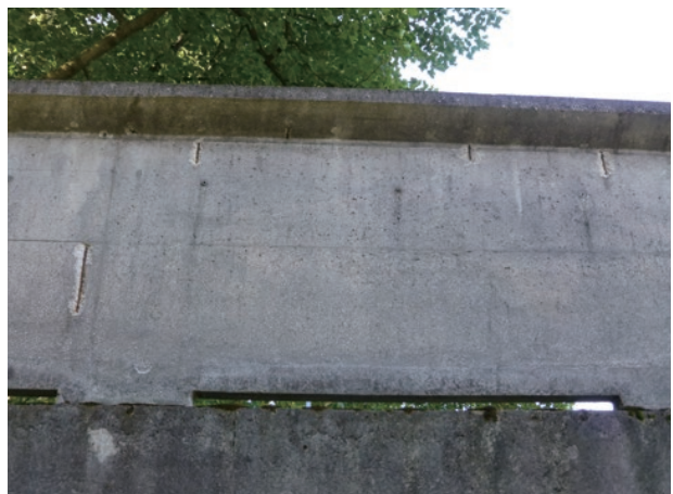
photo 68 Corroded steel bars (3)
