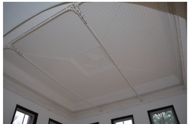
photo 29 Staircase, safety netting for ceiling plaster finish collapse
