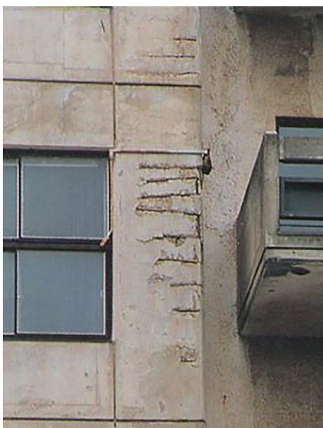
photo 3 Example of carbonation 3
