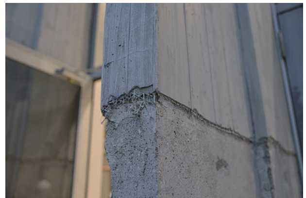
photo 6-4: Some of the finishing material was removed. (This view shows both the finishing material and the concrete underneath.)
