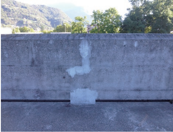
photo 63 Repaired concrete balustrade wall (the color of the concrete repair is conspicuously lighter)
