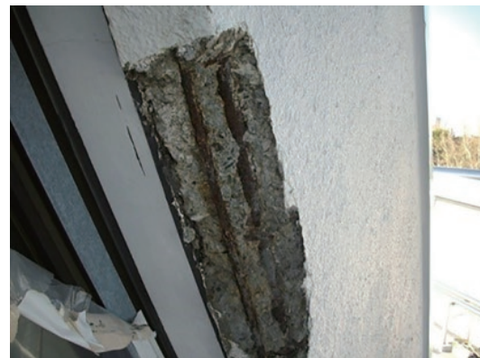
photo 4 Corrosion of the reinforced concrete around a skylight
