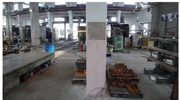
photo 7-6: Current appearance of a column undergoing re-alkalized in this project (photo provided by : West Japan Railway Company)
