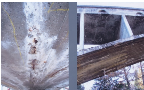
photo 43 Deteriorated Valterschiel Bridge before restoration (cited from a photograph of a signboard installed on site)
