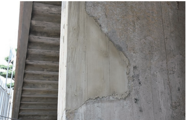
photo 5-13: A concrete surface from which the form has been removed after refurbishment using the injection method (photo provided by : The Japanese Association for Conservation of Architectural Monuments)
