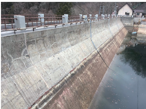
photo 3-7 : buttress frost damaged (photo provided by : Tokyo Electric Power Company Holdings, Incorporated)
