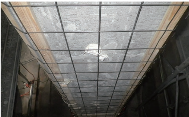
photo 7-2: Temporary anodes installed on the concrete surface (photo provided by : West Japan Railway Company)
