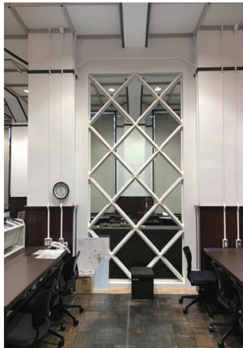
photo 10 Visible reinforcement at Former Institute of Public Health (Minato City Local History Museum)
