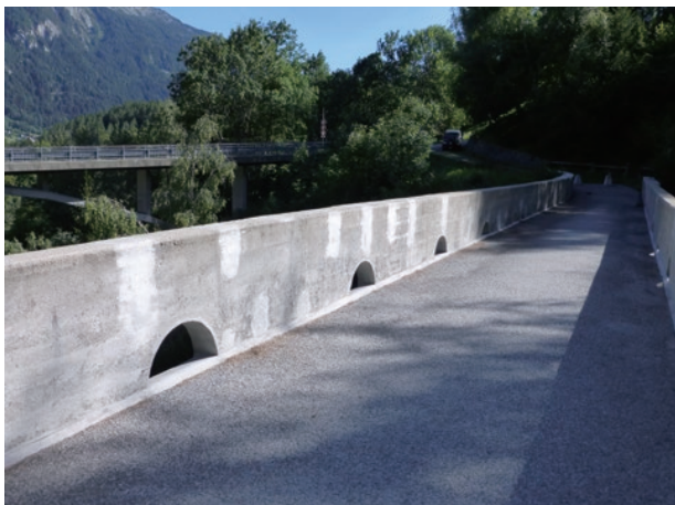
photo 46 Preventing rainwater that accumulates on the bridge surface from flowing out of the bridge
