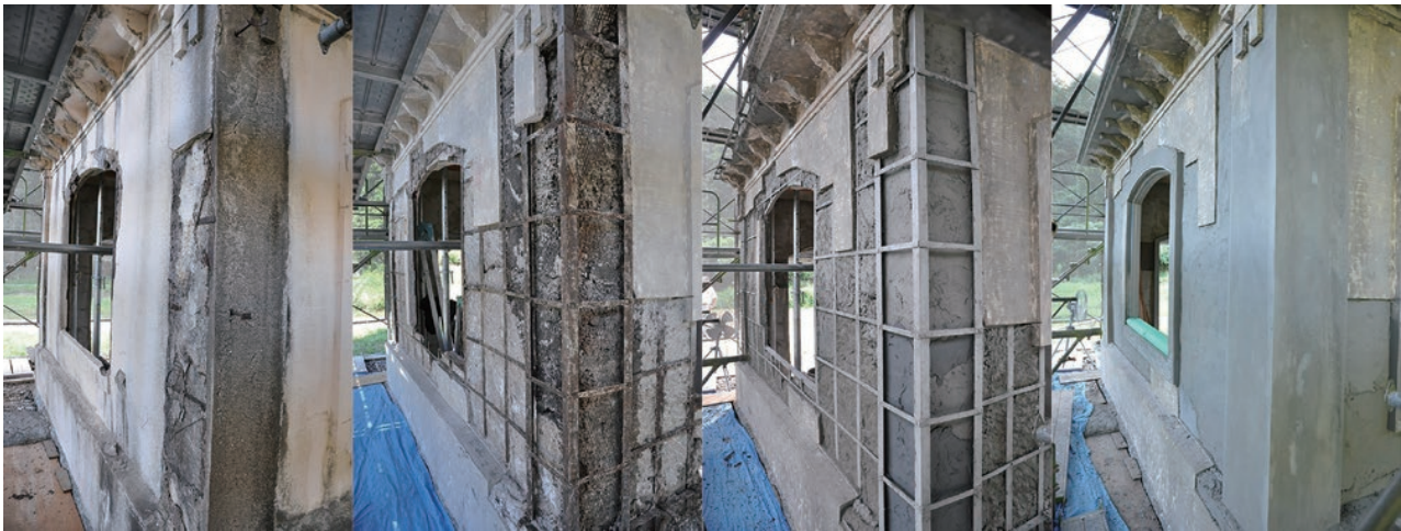
photos 4-4 to 4-7: Intake water control gate No.1 shed: ① before repair ② surface concrete was chipped away ③ rust-prevention of wire mesh and preparation of substrate ④ patch-repairing using mortar (reference: 『重要文化財 旧美歎水源地水道施設 保存修理工事報告書』、p.89)
