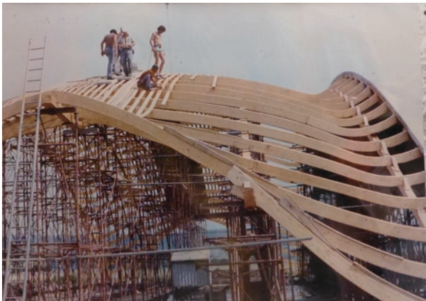
photo 53 Formwork scaffoldings being fabricated (cited from a photograph of a signboard installed on site)
