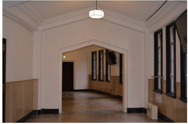
photo 27 Completed assembly hall corridor reinforcement wall. The opening was made with a pointed top to match the interior design
