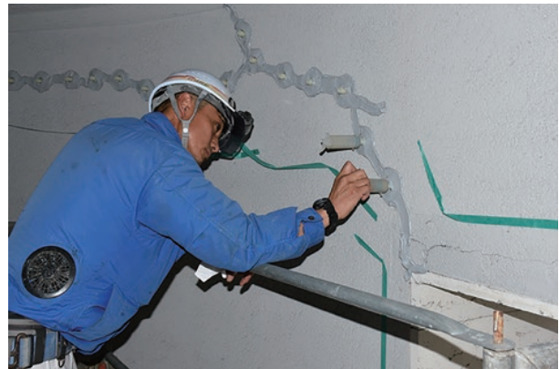
photo 5-7: Injecting cement slurry under low pressure (Internal wall) (photo provided by : The Japanese Association for Conservation of Architectural Monuments)
