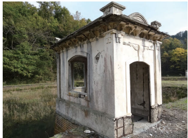
photo 2 Water control shed No. 2 before restoration. This was the most severely damaged of all wells.
