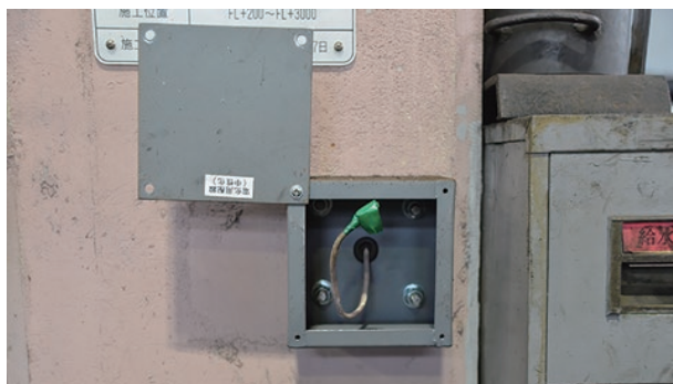
photo 7-9: Wiring for the internal electrodes left for monitoring purposes
