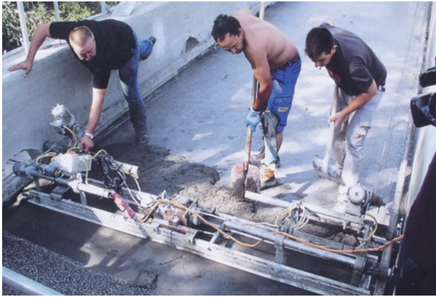
photo 44 Waterproofing using 2 layers of UHPRFC (cited from a photograph of a signboard installed on site)
