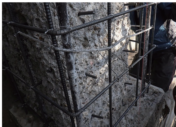
photo 3-9: Creation of framework of steel bars (photo provided by : Tokyo Electric Power Company Holdings, Incorporated)
