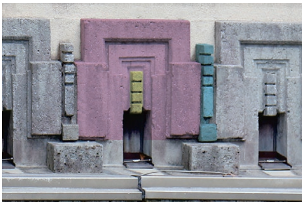
photo 1-2: Type A artificial-stone ornaments (with three parts reassembled) (red parts were newly placed in-situ) (photo provided by : Yodogawa Steel Works, Ltd.)
