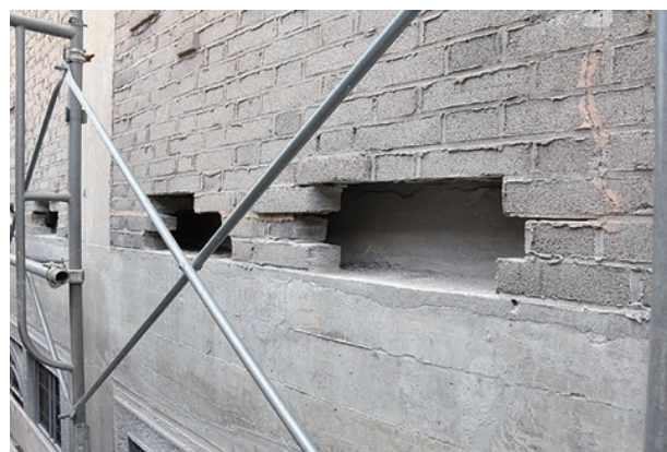
photo 5-2: External wall with double thickness (part of external wall mortared bricks removed) (photo provided by : The Japanese Association for Conservation of Architectural Monuments)
