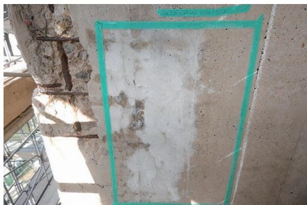
photo 2-10: Development of efflorescence: after the application of nitrite-based permeable rust-inhibitor+ silane-siloxane-based surface penetrant (photo provided by : The Japanese Association for Conservation of Architectural Monuments)
