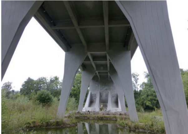
photo 25 Replication of the original surface pattern left by timber formwork on pier concrete surfaces
