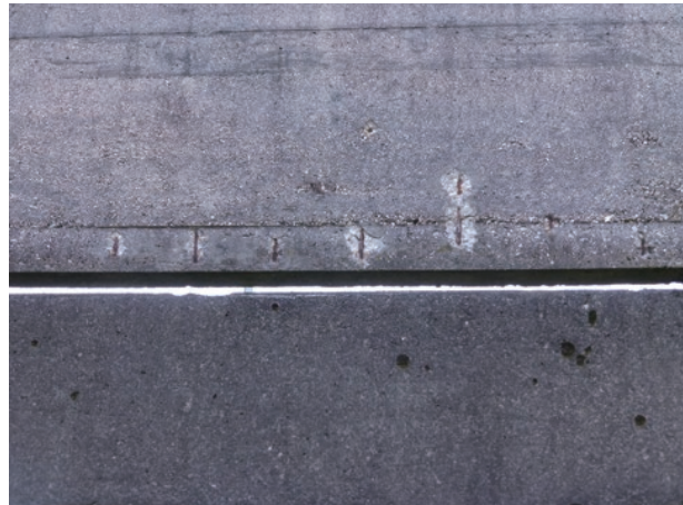
photo 67 Corroded steel bars (2)
