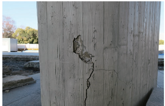
photo 6-3: Concrete pillar with a quasi-undressed finish, showing deterioration and damage
