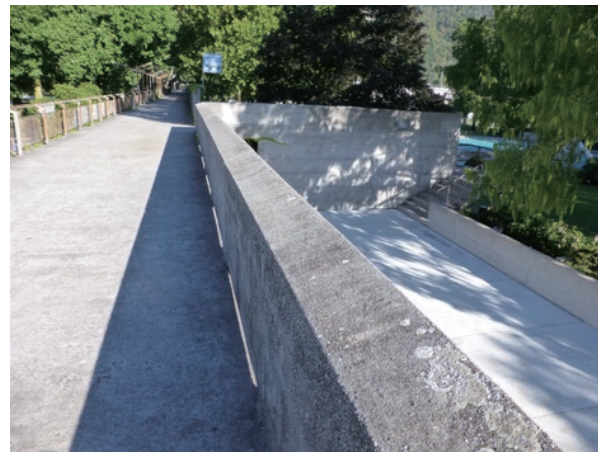
photo 61 Installation of a water-resistant layer made by spraying concrete over the surface of the concrete wall balustrade (the color of the repaired areas goes well with the color of the surroundings)
