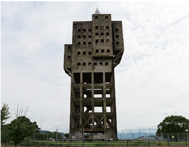
photo 2-1: Exterior view of the Former Shime Coal Mine Shaft Tower before restoration
