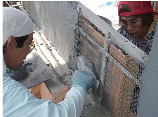
photo 4-1: Steel-framed building whose exterior walls were finished by mortar applied over a steel wire mesh (reference : 『重要文化財 旧美敷水源地下水道施設 保存修理工事報告書』、p.87)
