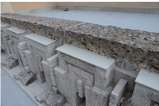
photo 1-3: Galvalume steel sheets on top of ornaments to serve as a form of eaves.
