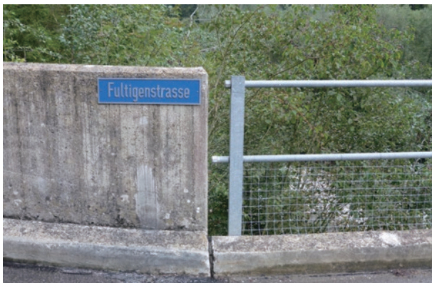
photo 5 A water repellent was applied to the surfaces of the concrete balustrade and wheel guard.
