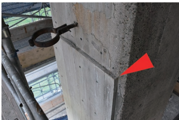
photo 2-9: New concrete was placed to areas whose thickness of covering concrete was insufficient (increased thickness indicated by a red arrow) (photo provided by : The Japanese Association for Conservation of Architectural Monuments)
