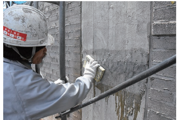
photo 5-8: Decorative coat being applied to a repaired area of the concrete (photo provided by : The Japanese Association for Conservation of Architectural Monuments)
