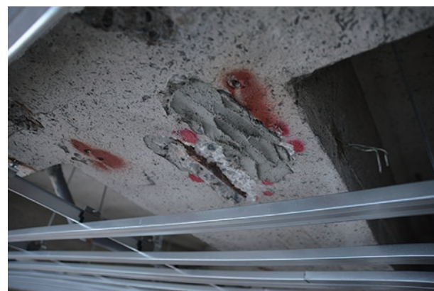
photo 6-7: Areas where repaired parts could be hidden using a finishing material were treated in such a way that the repaired area could be clearly identified
