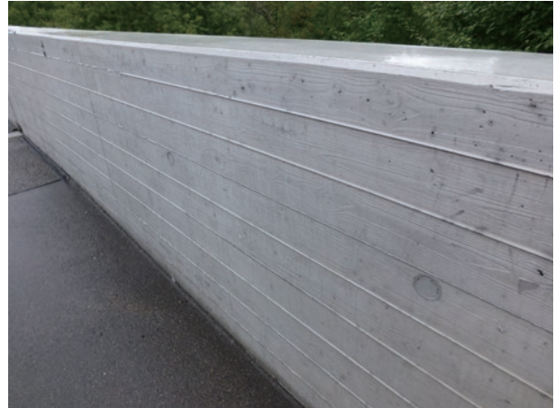
photo 26 Replication of the original surface pattern left by timber formwork on balustrade concrete surfaces
