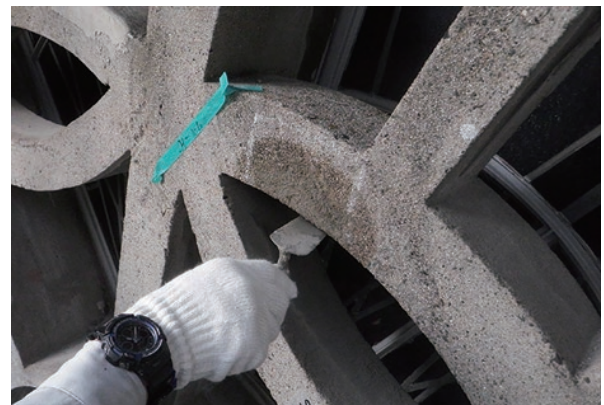
photo 5-9: Precast concrete area being repaired (photo provided by : The Japanese Association for Conservation of Architectural Monuments)
