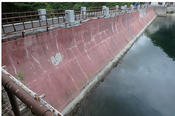
photo 3-2: The protective coating of the dam's upstream face peeling away (photo provided by : Tokyo Electric Power Company Holdings, Incorporated)
