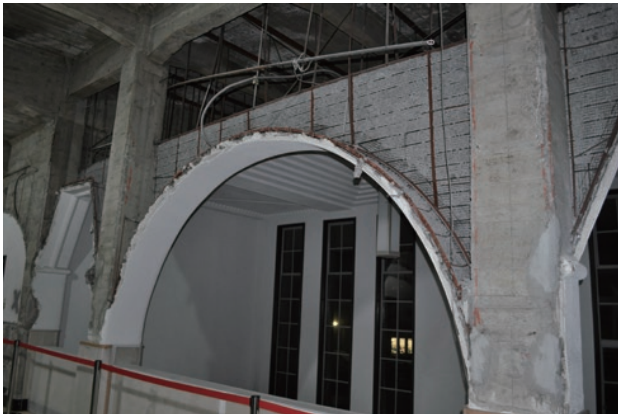
photo 23 Before installation of reinforced concrete anti-seismic wall. Removal of decorative mortared arch of lath substrate
