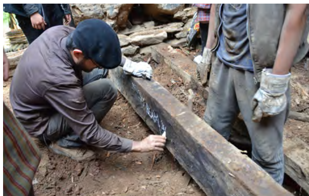
Temporary marking collapsed wooden members with chalk
