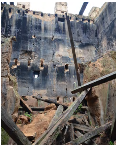
Inside view from the west showing the collapsed central section of the partition rammed earth wall
