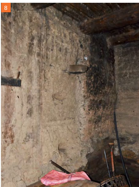
8 Traces of the former partition wall on the attached part's south wall of the ground floor
