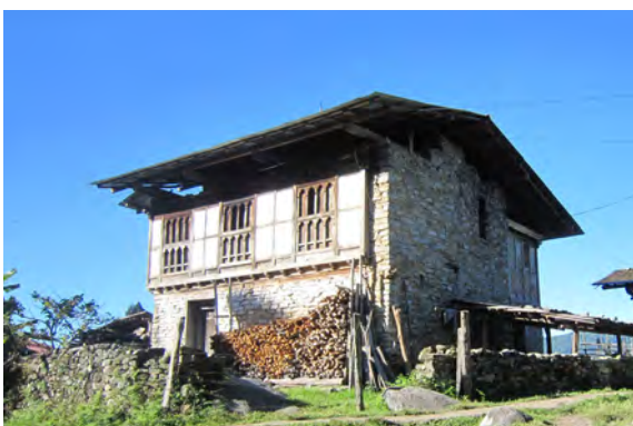
Traditional house with masonry walls and a timber frame (Buli, Zhemgang Dzongkhag)
