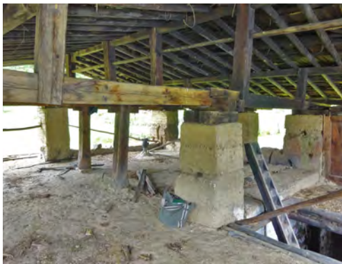
Attic space (rammed earth structure shows the four corners of original form)
