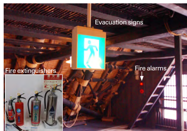
Fire prevention equipment of traditional houses in Shirakawa-mura
