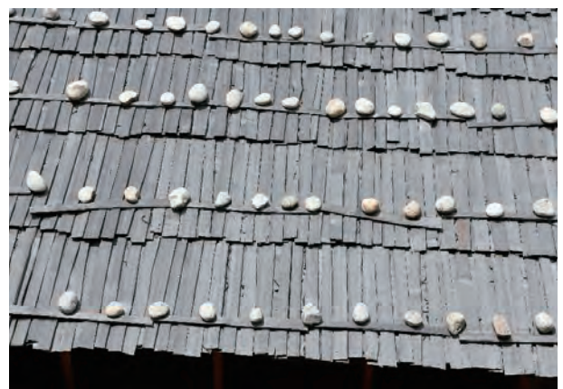
An example of a shingle roof combining traditional and modern construction methods (renovated traditional house near Paro Airport)
