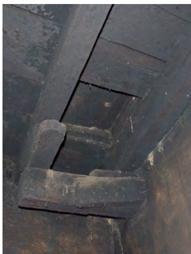
Bracket beam of the overhanging section shown in the living room of the first floor
