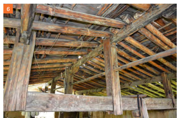
4 Rabsel window of the room on the south side of the first floor 5 Room on the north side of the first floor 6 Roof structure
