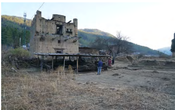
Lham Pelzom House in January 2019 after salvaging, sorting and storing all collapsed wooden members in the temporary shelter
