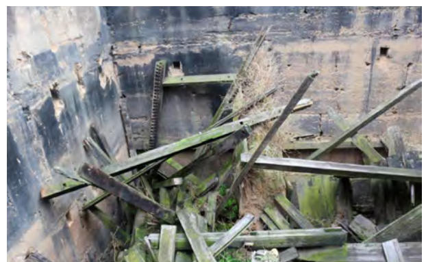
Inside view from the north showing as-found condition of collapsed wooden members
