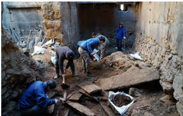
Removing the earth to salvage buried members in the east side of the building
