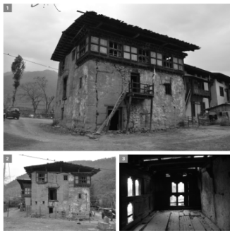
1 Whole view of the front side 2 Evidence of rammed earth expansion shown on the sidewall 3 Living room on the front side of the second floor
