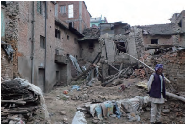
Fig. 4-2-10 The collapsed house at the rear side of N04
