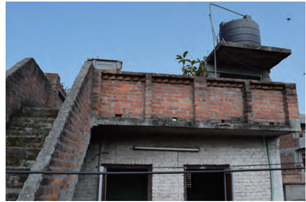
Fig. 4-2-11 Water storage tank placed on the roof top (N13)
