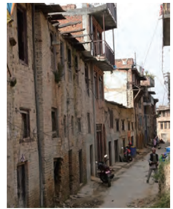
Fig. 4-1-8 Half collapsed traditionally constructed buildings
