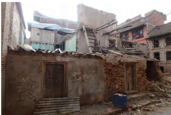
Fig. 4-2-23 Heavy damage of the building Type AB
