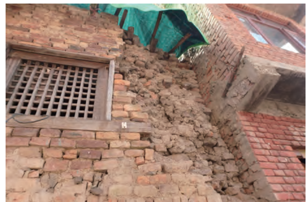
Fig. 4-2-13 Damage of a brick wall after the disaster, with peeling off of surface brick
