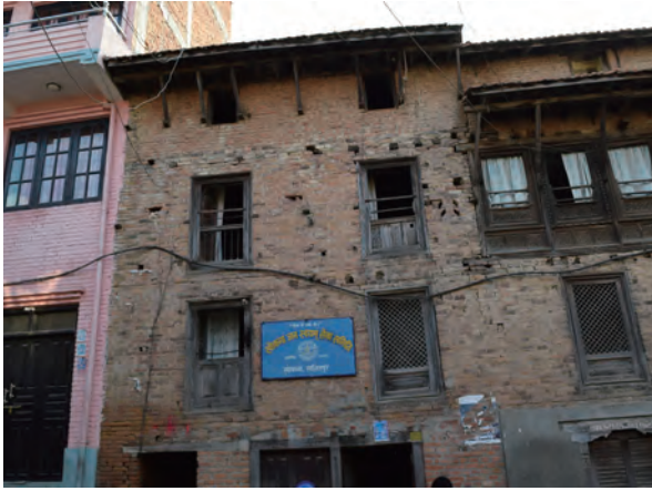
Fig. 4-2-1 House extended on the 3rd floor (S16). Roof and struts are relocated to one floor higher up. The trace of the past supporting beams is left on the façade.
