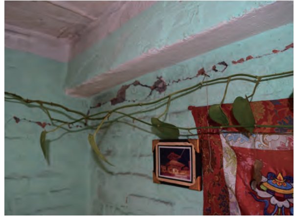
Fig. 4-2-2 Cracks over the wall under the beam of the extended floor.
