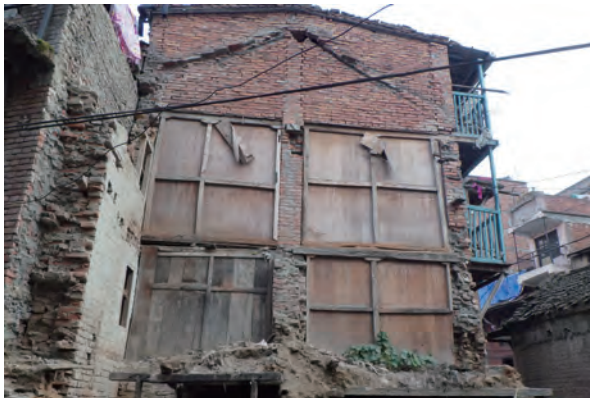
Fig. 4-2-8 Example of damaged houses (N00) neighboring the one with blue balcony (N01)
