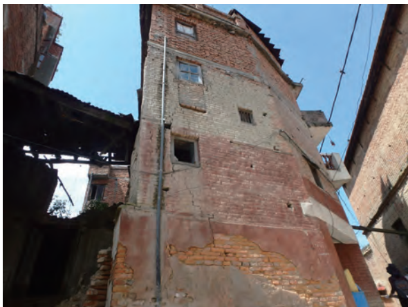
Fig. 4-2-4 Example extension of reinforced concrete on the houses (An example from outside of the investigated site)
