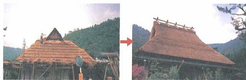
Repair of a historic building (vernacular house with thatched roof) at Kita, Miyama-cho
