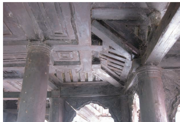
Ph.33 Depression at the end of the lower beams of a tower (Bagaya monastery, Innwa)
