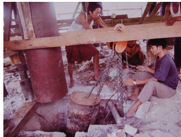
Ph.19 Cutting the bottom part of a pillar (during restoration of a Zayat in Mandalay)
