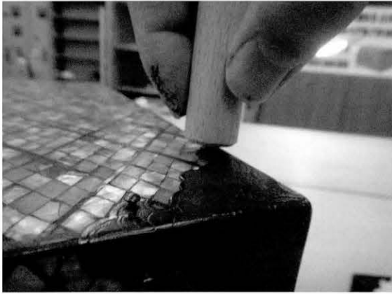
Fig. 5.19 隅金具と取り付け 修復中 Attaching a corner metal fitting, during restoration
