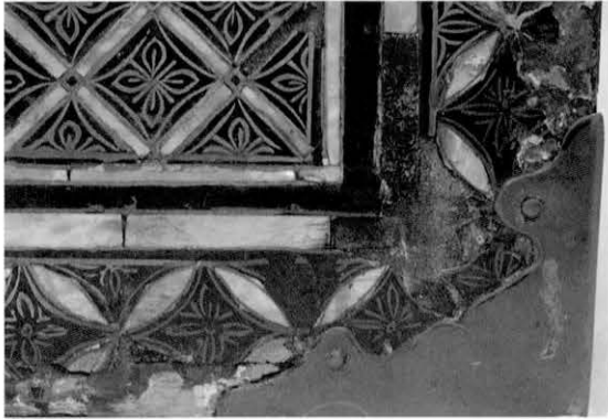
金具周辺部分の損傷 Damage around a metal fitting, 2006
