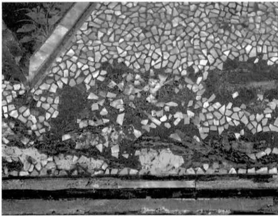
螺鈿の剥落 Missing raden shell pieces, 2006
