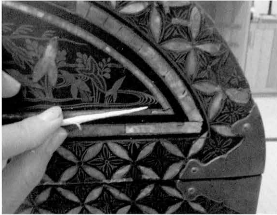
漆塗膜の劣化 後補塗料の劣化 Deterioration of ursuhi coating film, deterioration of coating material from past restorations, 2006
