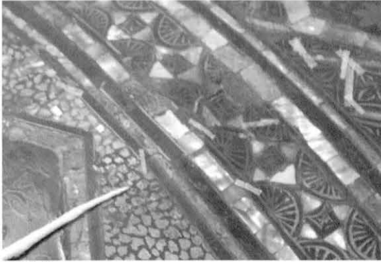
後補塗料 Coating material from past restorations, 2006
