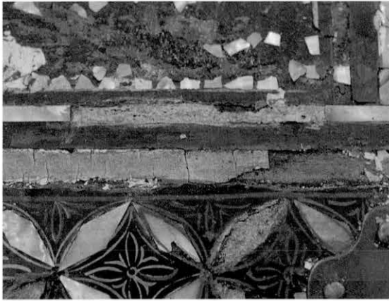
後補材料の剥落 Loss of restoration material from past restorations, 2006
