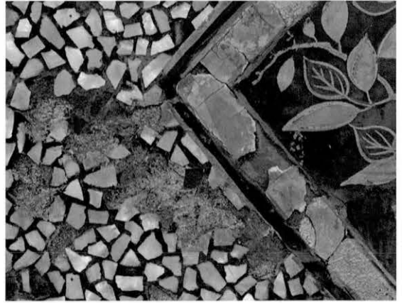
後補材料の剥落 Loss of restoration material from past restorations, 2006
