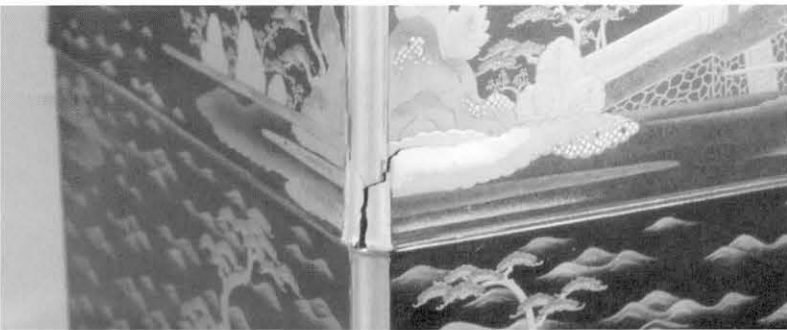
図7 身の上段角 亀裂部分 Corner of the upper tier of the body seen from the outside, cracked portion
