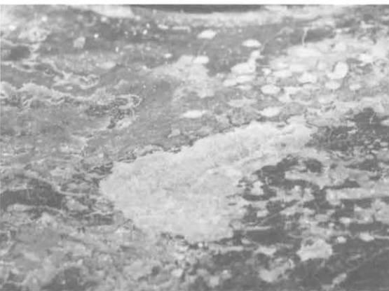
図14 修理前 肩の塗膜欠損部と付着した汚れ Shoulder before restoration, part with missing coating film and dirt
