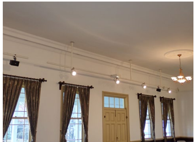
Photo Lighting equipments and sound system in the main hall
