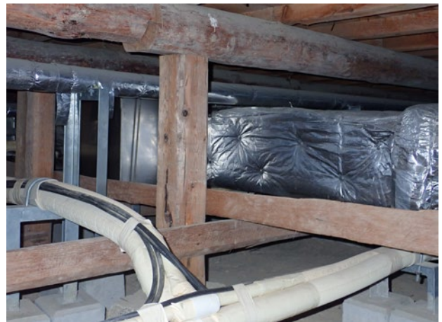
Photo Air conditioner duct under the main hall
