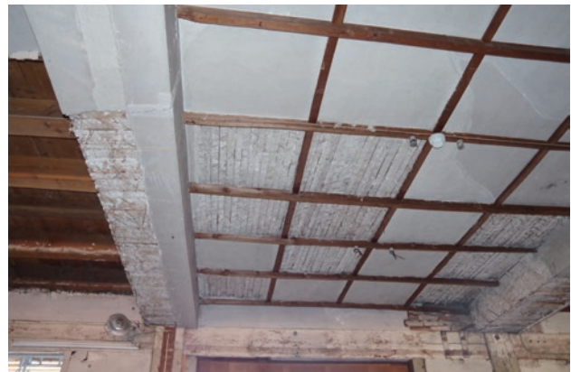
Photo 5 West Cocoon Warehouse, first floor, wooden lath underneath of the ceiling, before preservation and repair work
