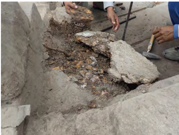
Figure 9.2.28 Fragile laterite blocks deteriorated by the penetration of tree roots
