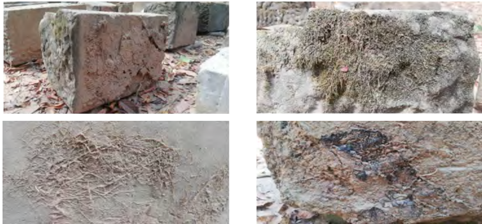
Figure 9.1.1 Examples of stone damage
