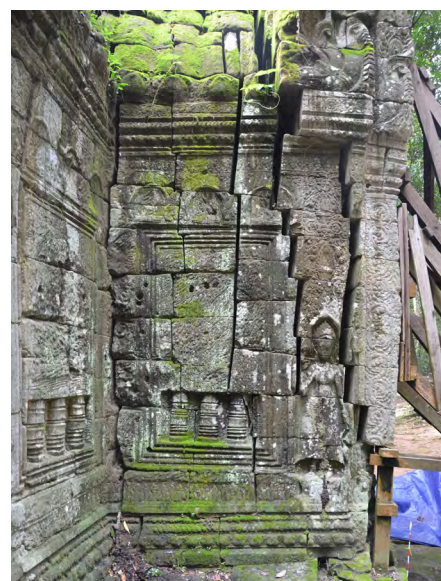
Figure 8.1.2 Continuous open joints in the vicinity of an external corner
