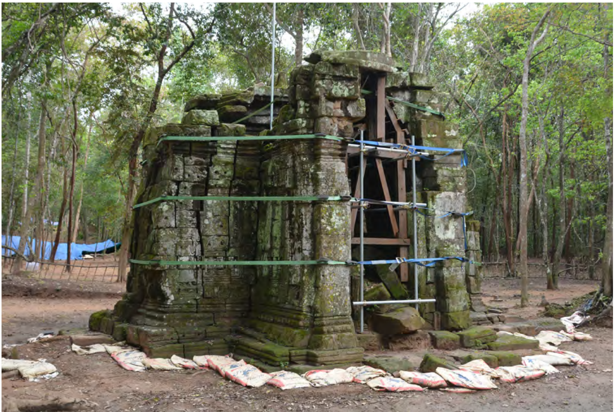
Northwest elevation before dismantlement (after the removal of the scattered stones) in September, 2019
