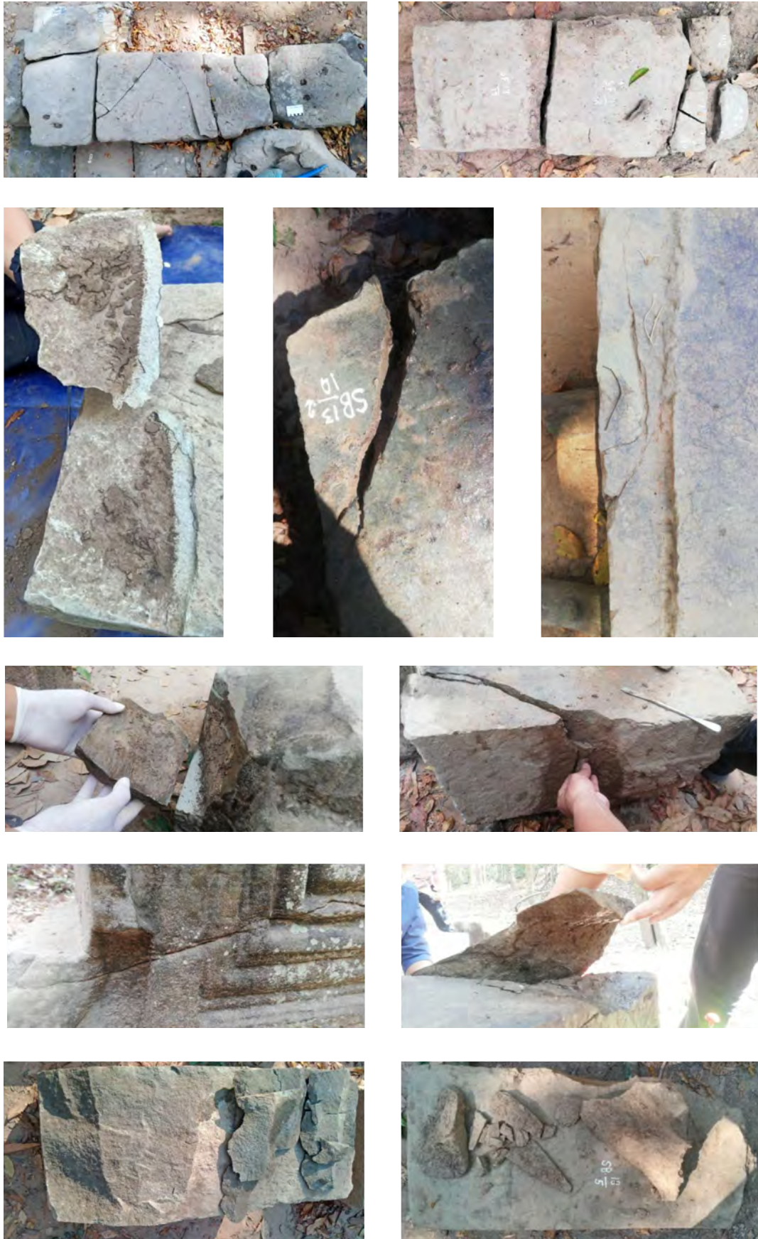
Figure 9.1.3 Examples of stone cracks
