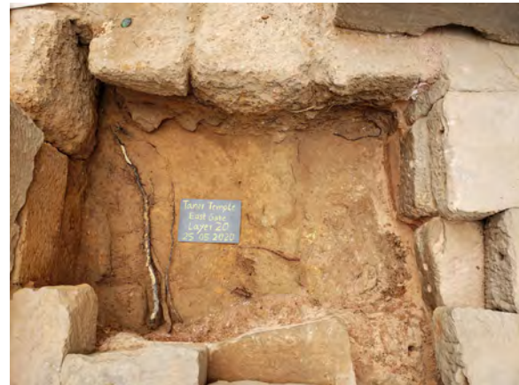
Figure 9.2.35 Condition of the compacted soil below the deteriorated substrate laterite in the east wing
