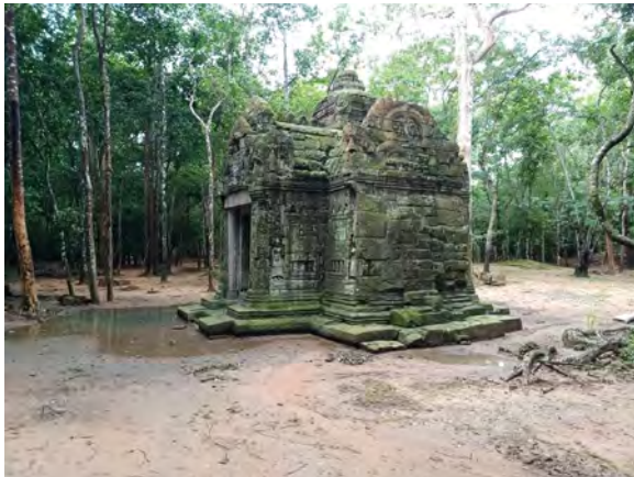
Figure 9.3.7 Unresolved water stagnation on the eastern side of the East Gate (August 2022)
