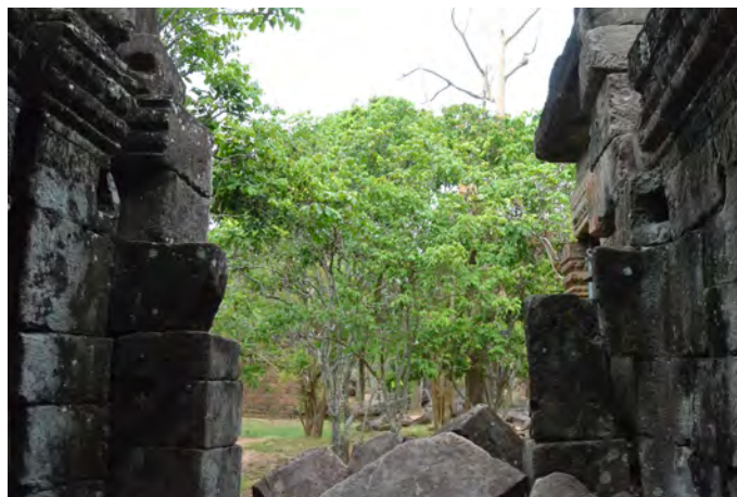
Figure 3.2.52 Traces of the wooden members at the west entrance, Banteay Thom Temple
