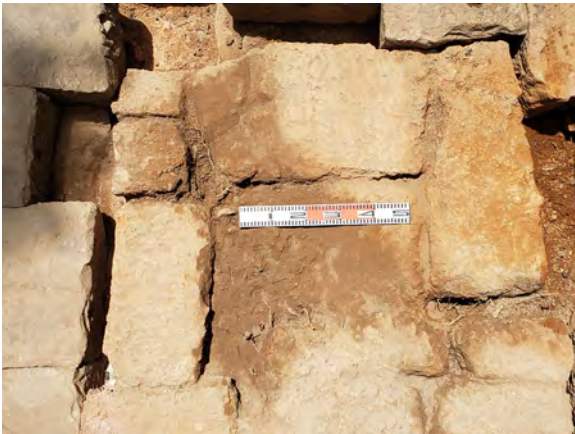
Figure 9.2.34 Deteriorated substrate laterite in the east wing
