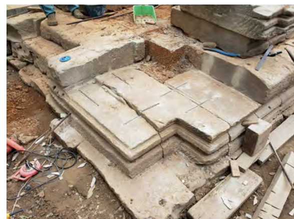
Figure 9.2.55 Stainless steel clamps inserted at the northeast corner of the east wing to prevent sandstone displacement
