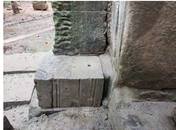
Figure 9.2.69 Base of the new colonette, shaped by following the traces on the adjacent stone surface at the northwest corner
