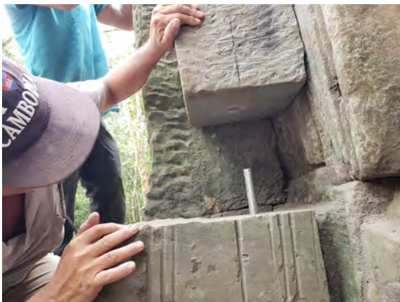
Figure 9.2.70 Stainless shear connector inserted at the bottom of the new colonette at the northwest corner
