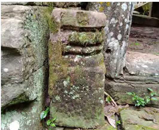
Figure 5.2.22 Bottom of the colonette that stands at the West Gate's western entrance
