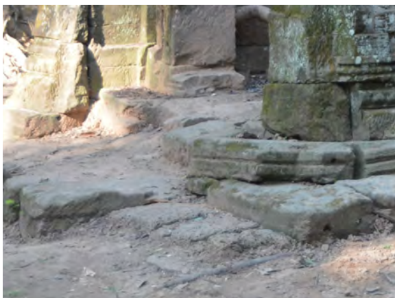
Figure11.1.1 Laterite members of the East Gate base structure at the southwest corner
