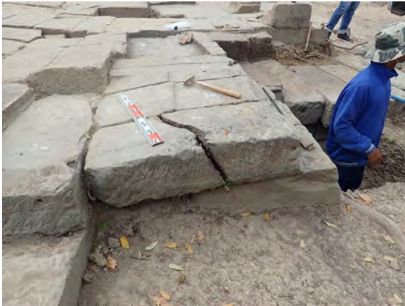
Figure 9.2.26 Outflow of infill soil that caused the brake of exterior sandstone
