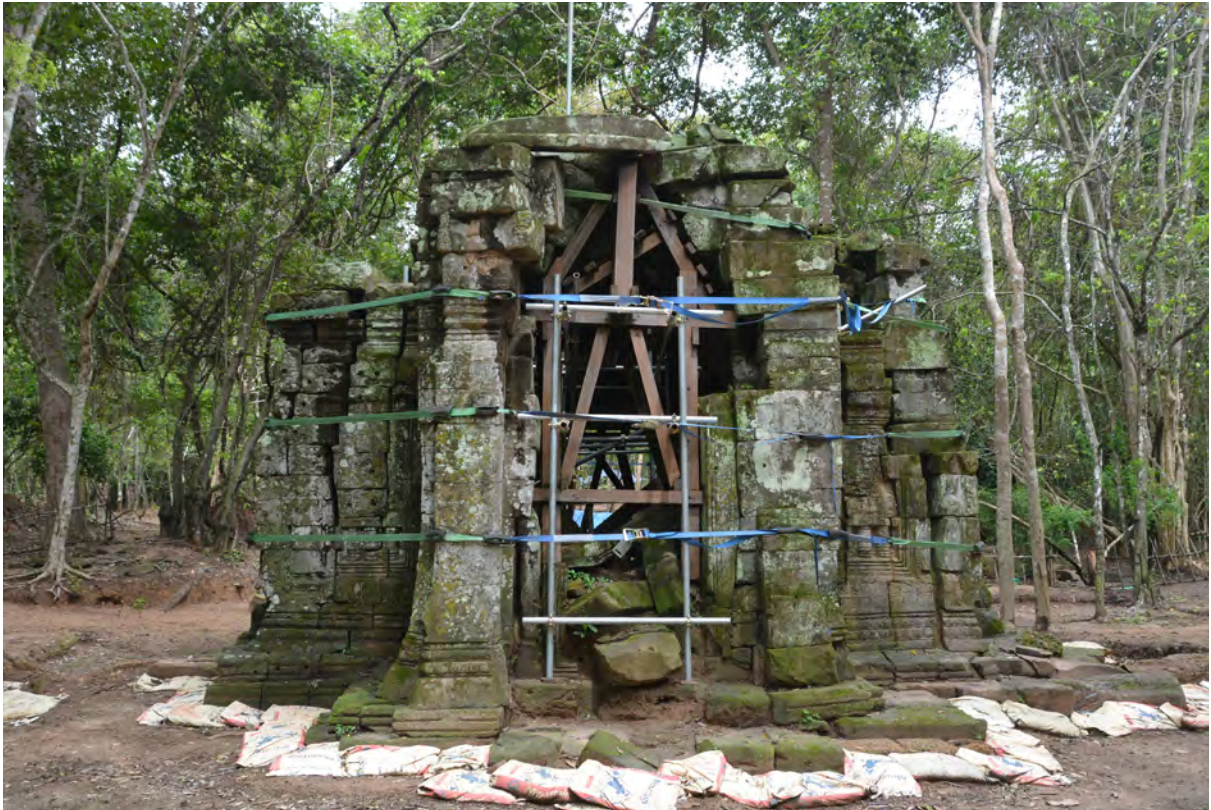
West elevation before dismantlement (after removal of the scattered stones) in September, 2019
