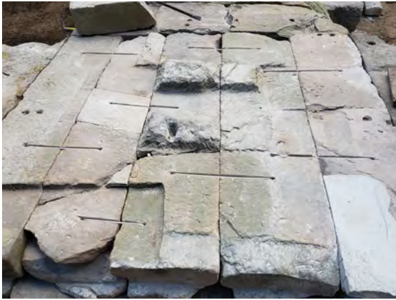
Figure 9.2.88 Consolidation of the central part of the roof using long stainless steel clamps
