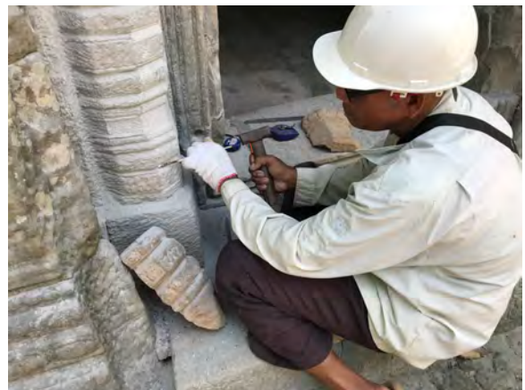
Figure 9.2.105 Engraving the colonette's new stones, with reference to a fragment of the original colonette
