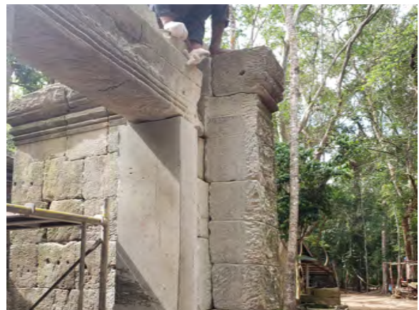
Figure 5.2.29 Traces on the north side wall show no support for the northern edge of the eastern lintel on the wall
