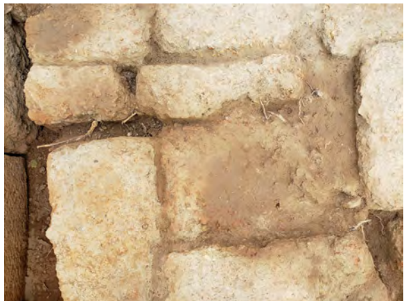
Figure 9.2.29 Situation of the penetration of tree roots
