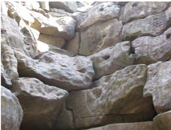
Figure 9.2.96 Minor defects at the roof's northwest corner
