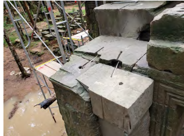
Figure 9.2.73 Use of clamps to consolidate the new colonette, the pilaster and the wall
