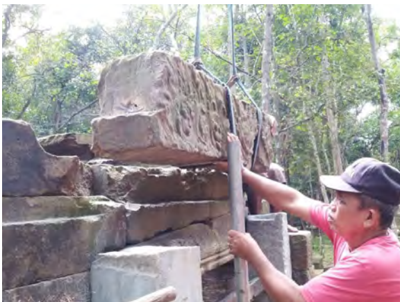
Figure 5.2.28 Tiered joints between the lintel and the upper door frame, with no mortise hole on the bottom surface of the lintel where the colonette attaches
