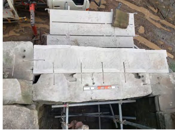
Figure 9.2.77 Stainless steel clamps used to connect the lintel and the stone from the rear
