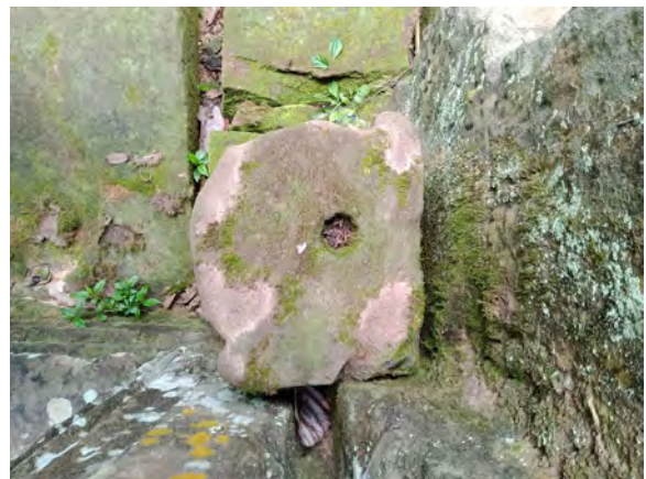
Figure 5.2.23 Smoothed upper surface with a hole in the bottom of the colonette that stands at the West Gate's western entrance
