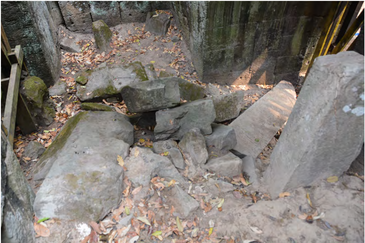
Collapsed stones inside the East Gate in March, 2019
