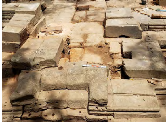
Figure 9.2.33 Deteriorated substrate laterite in the east wing
