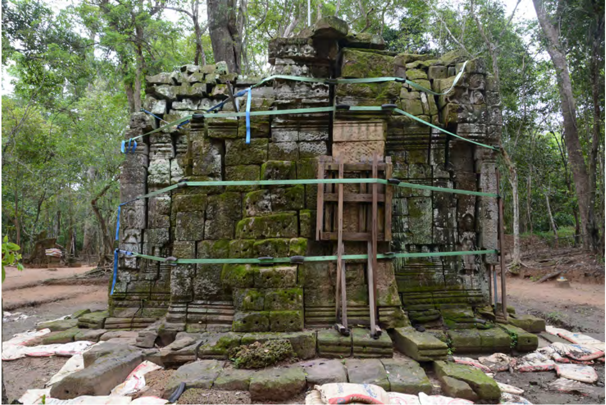
South elevation before dismantlement (after removal of the scattered stones) in September, 2019
