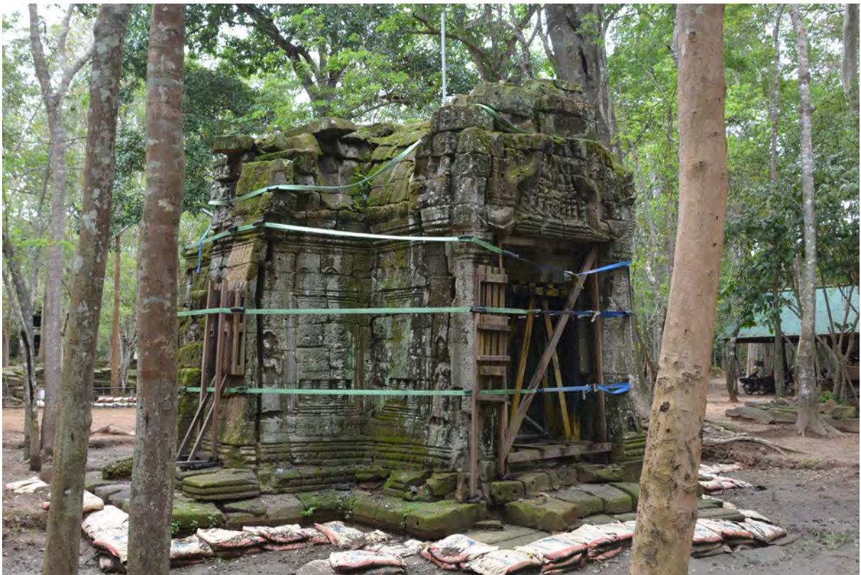
Southeast elevation before dismantlement (after removal of the scattered stones) in September, 2019
