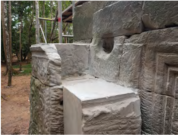
Figure 9.2.72 Cutting the deteriorated part of the pilaster to consolidate with the new colonette using a clamp
