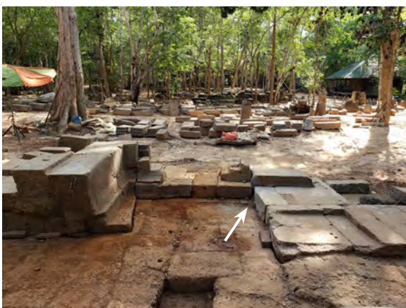
Figure 9.2.54 Gap that occurred between exterior sandstones in the northwest corner of the west wing
