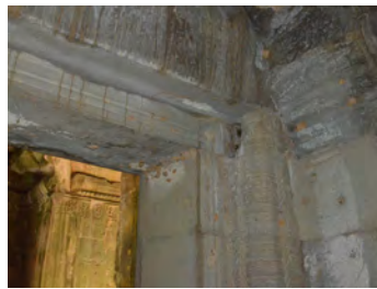
Figure 3.2.48 A trace at the entrance of the side chamber, Preah Khan Temple
