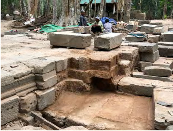
Figure 9.2.32 New laterite block inserted in the southeast part of the east wing
