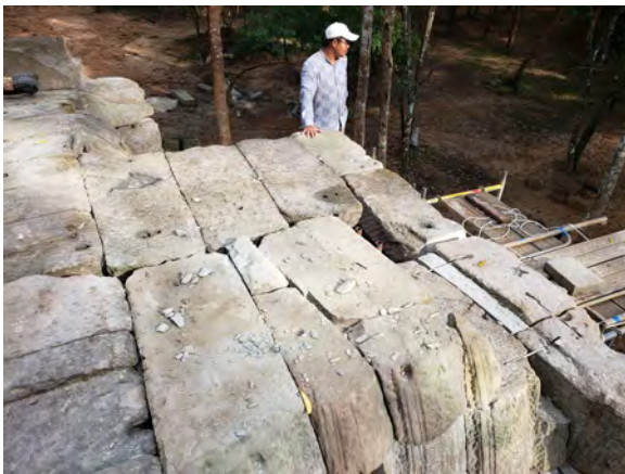
Figure 9.2.84 Layer 01's top surface and the use of stainless steel clamps at the pediment
