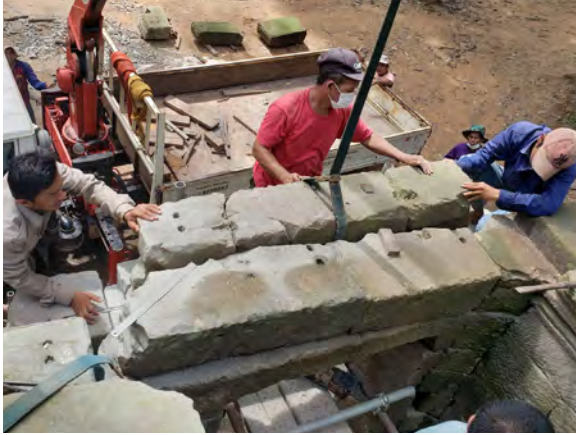
Figure 5.2.30 Upper surface of the lintel and the door frame, fastened using H-shaped clamps
