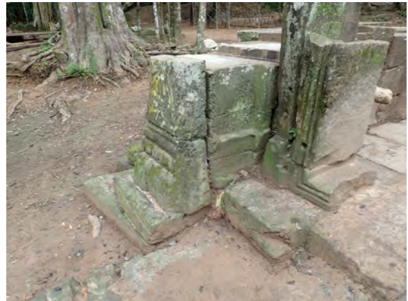
Figure 5.2.27 Smoothed upper surface without mortise in the northwestern corner where the colonette stands
