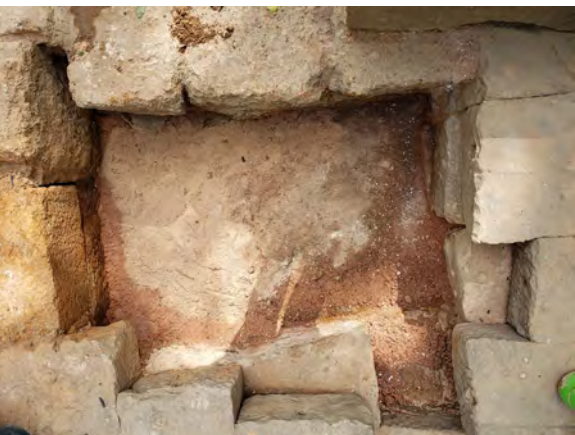
Figure 9.2.36 New lime mortar compacted on Layer 20's top surface before insertion of new laterite
